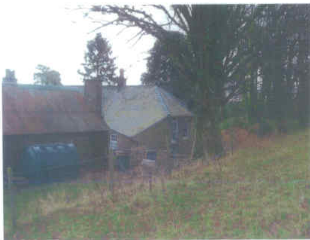
Fencing obstructing access into Tyle Gwyn Farm
